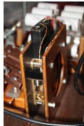
Figure 4.27: The power supply of the fan.
