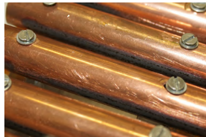
Figure 4.24: Heavy corrosion between the copper tubes.
